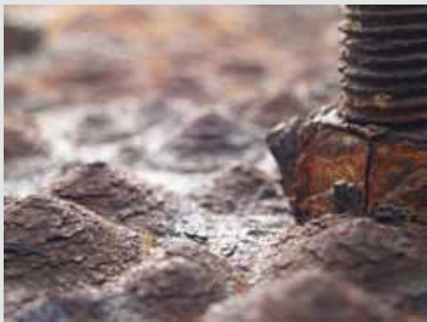
Prevent this! Corrosion due to "wrong" material
